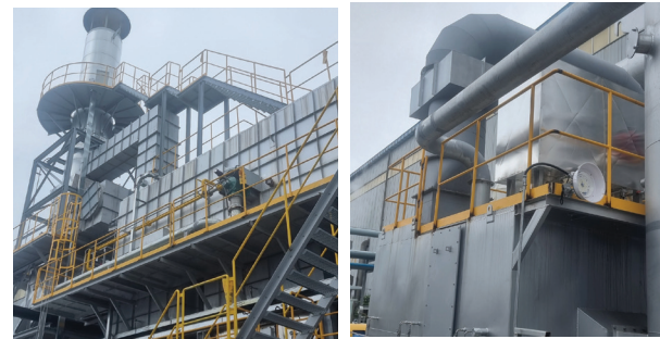
New RTO system equipment at SeAH Coated Metal
